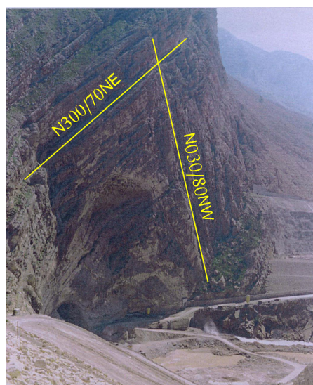
Fig.8. Several joint sets cut the Asmari limestone at the site. The rock mass is cut by two major sets of joints. One major joint set strikes 030 and dips 80 degree NW. The other major joints set strike 300 degree and dips 70 degree NE.
